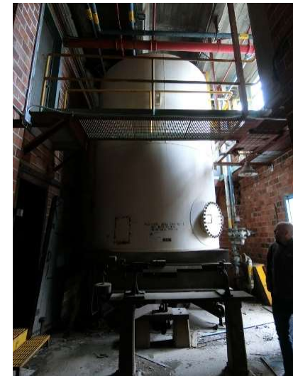
Existing denaturing tank
