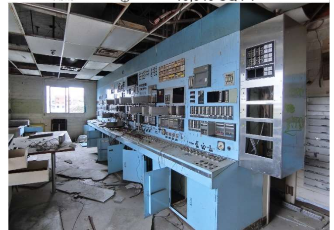
The Control Panel
