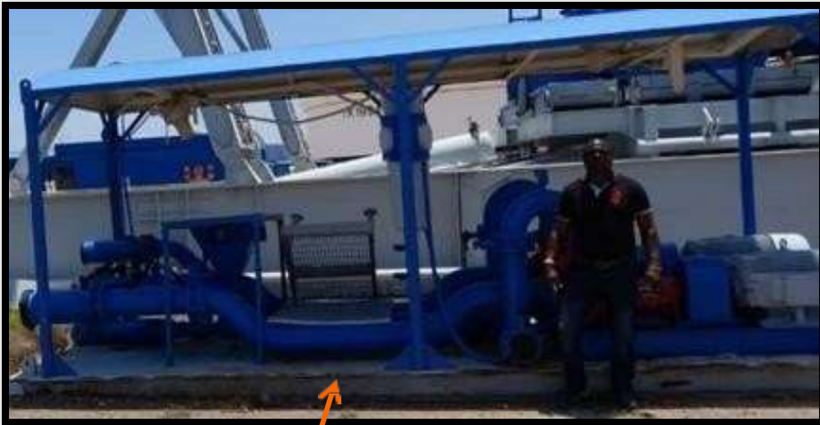
Mud Transfer Unit
