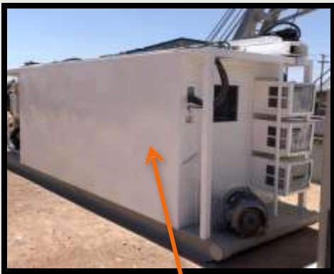
CANRIG CONTROL HOUSE
