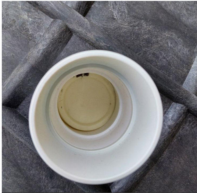
Cable outlet pictured
