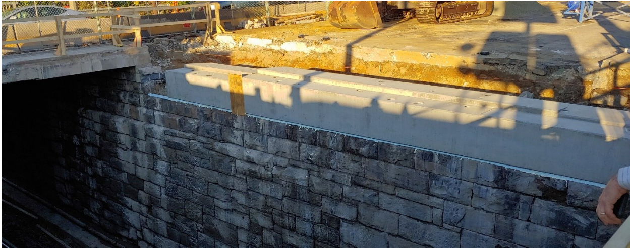
Photo: Existing Masonry Abutments with new Precast Abutment Cap, W. Girard Ave over CSX RR, Philadelphia, PA
