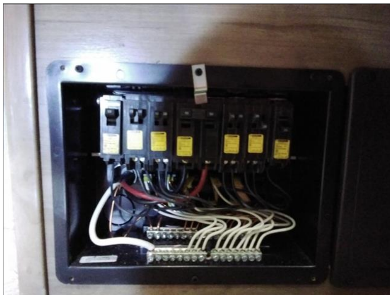
fuse panel 120 VAC
