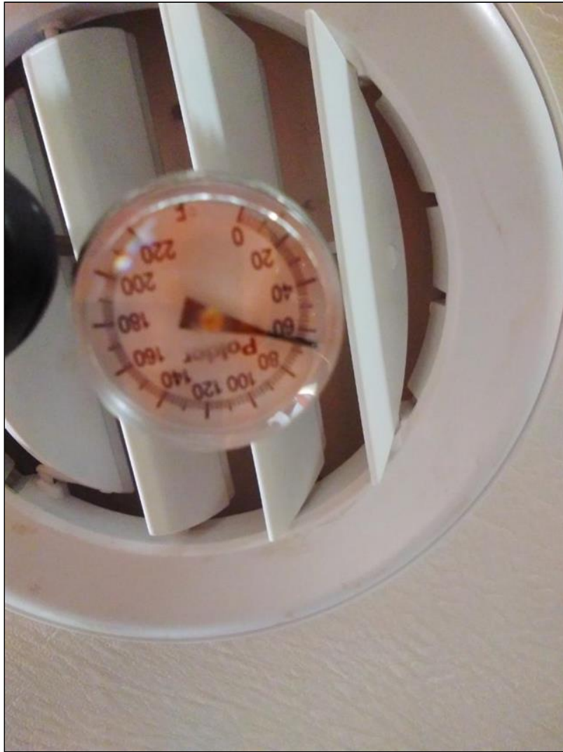
cooling vent photo
