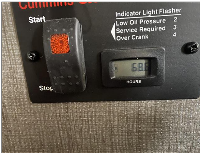
Generator interior panel
