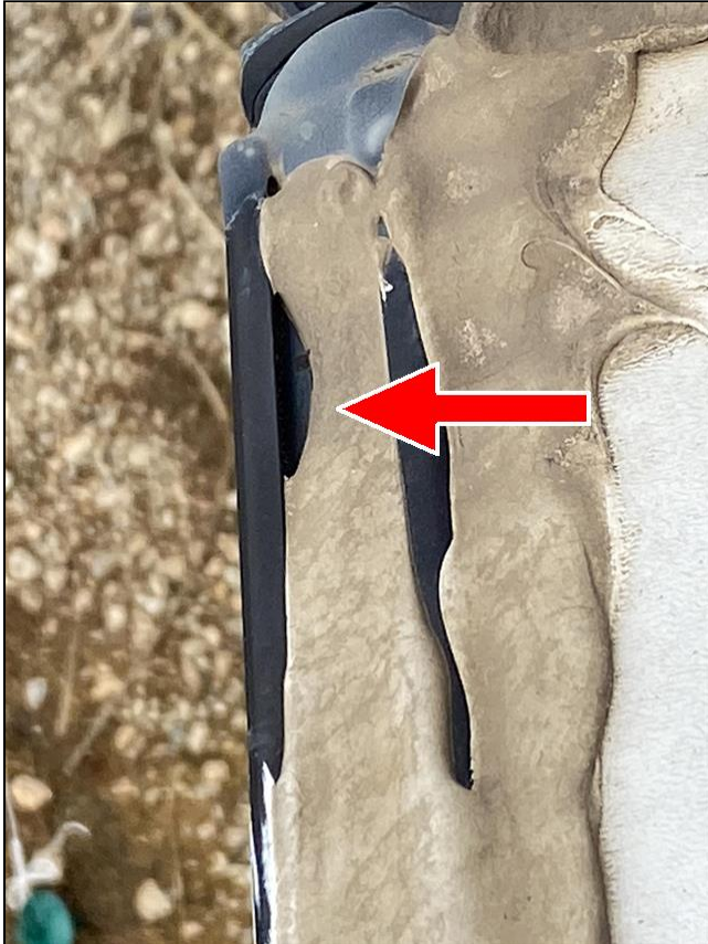
Streetside rear cap seal
