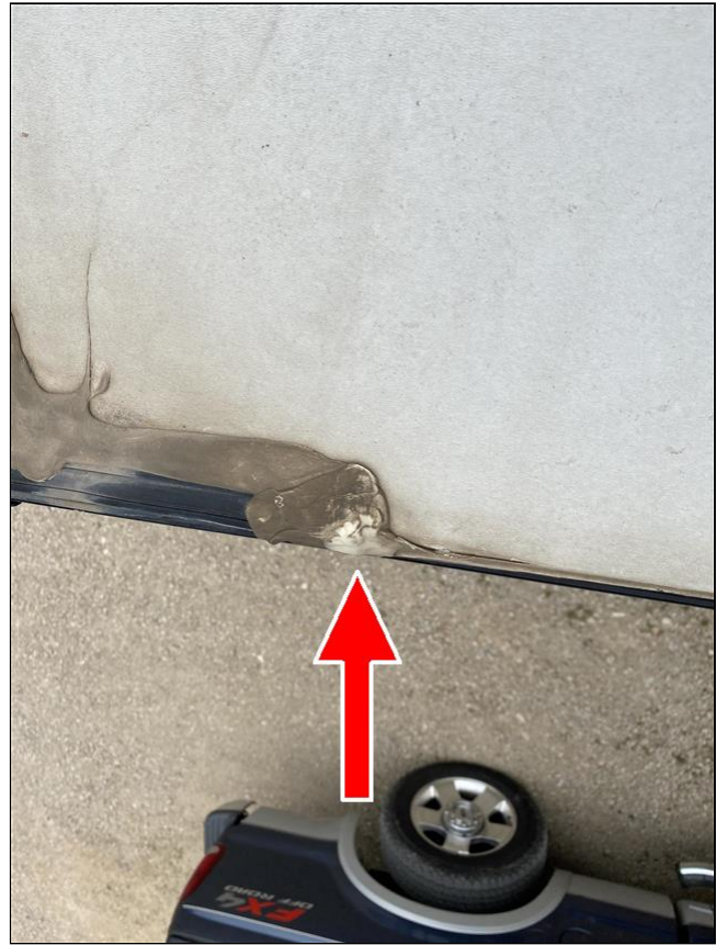
Peeling sealant on street side front cap seal
