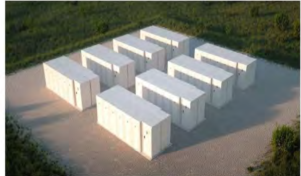
Typical Containerized Battery Modules
