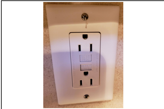
Electrical Outlets are GFCI
