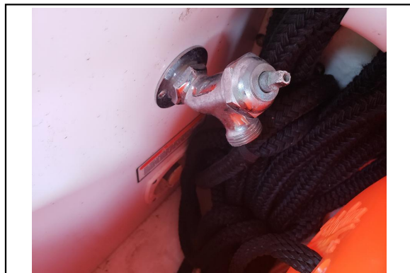
Water City Handle Missing
