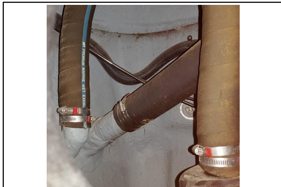
Exhaust Hoses Double Clamped
