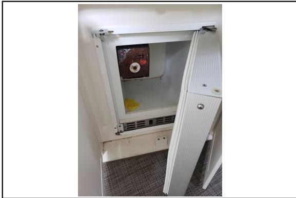
Cockpit Galley Ice Maker Does Not Work
