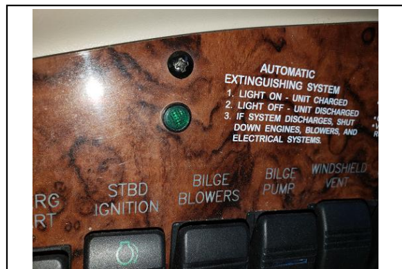
Helm Fire Extinguisher Shows Charged
