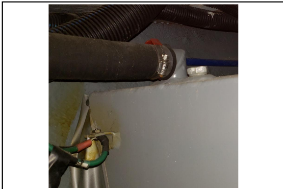
Fuel Tank Inlet Hose Double Clamped
