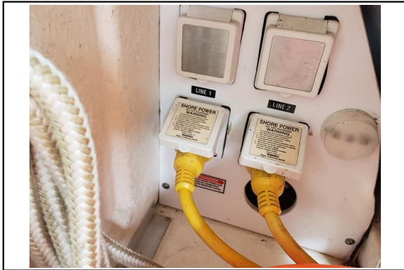
Shore Power Cables Two
