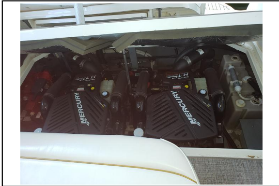
Engine Compartment Overview
