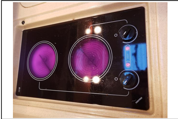
Galley Stove on Generator
