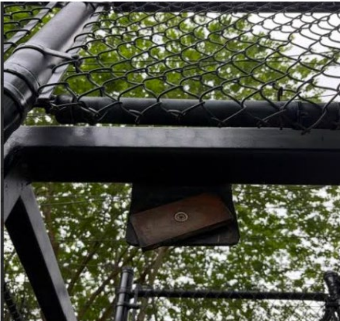
Court Entrance Door – Magnet on door shifting down
