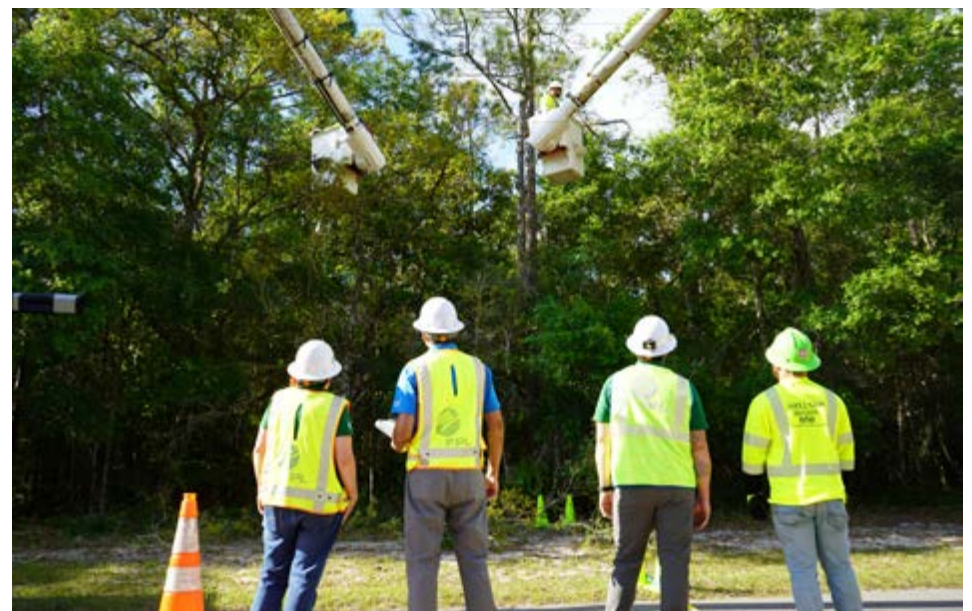
One of the major causes of power outages is vegetation, so FPL is trimming trees and other growth from 268 miles of power lines. Image provided.
