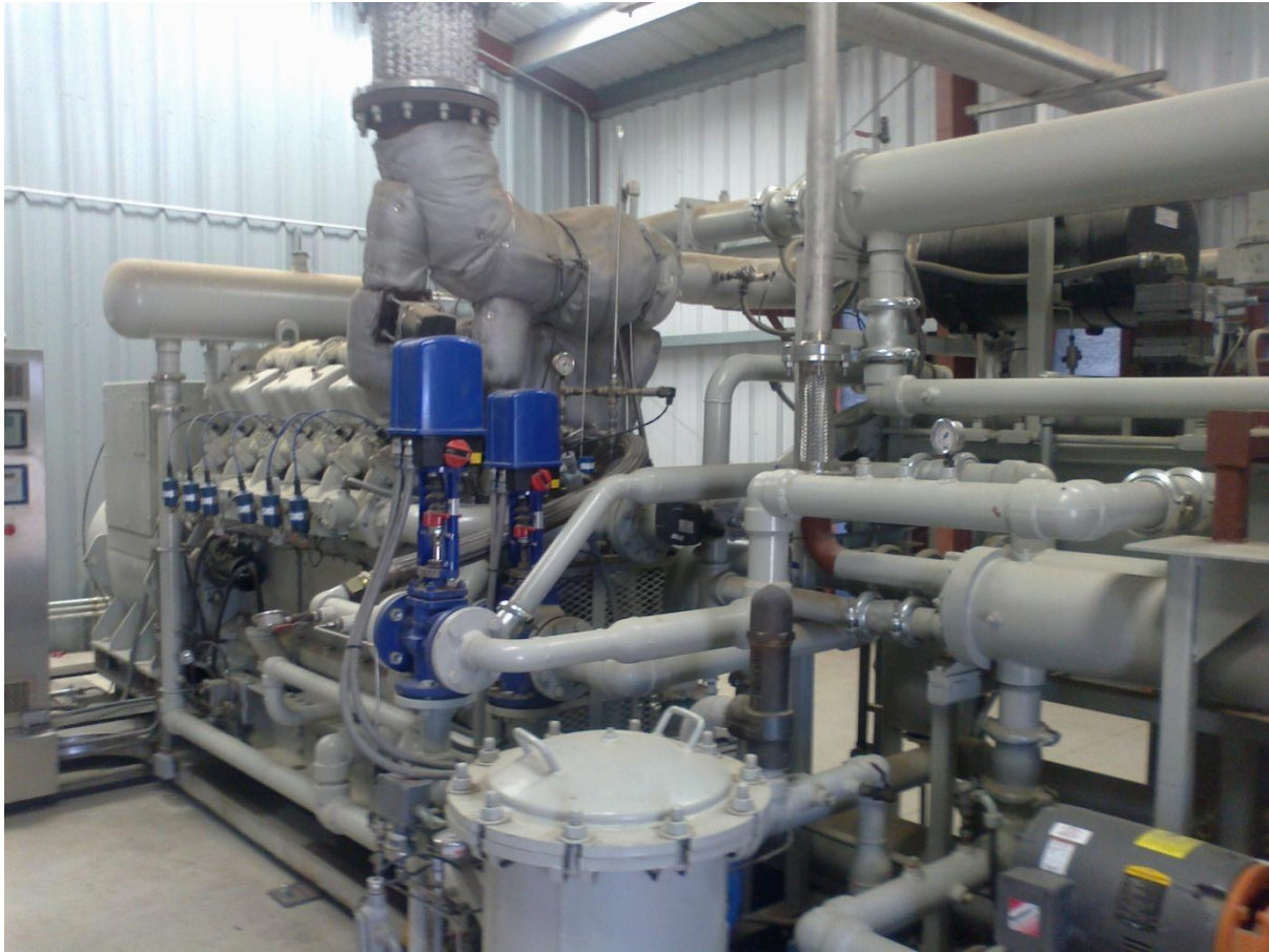
Figure 2 Bio digester generator Stockdale Road dairy
