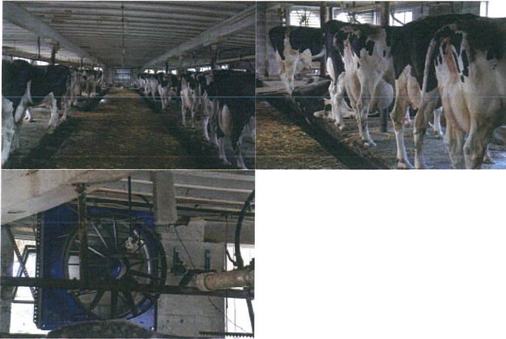
Plate 12-14: Slightly different ventilation system which was newly added
