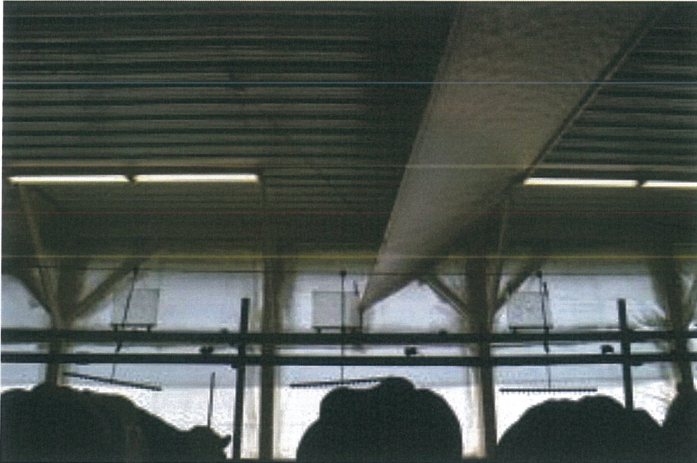
Plate 23: Baffles which drop cool air onto the backs of the cows
