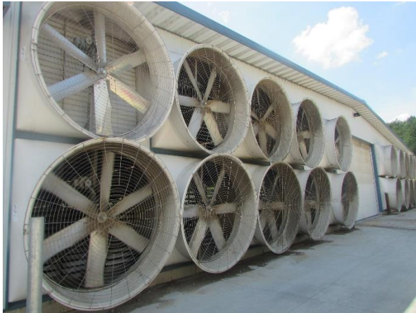
Fan system at Kutz Dairy
