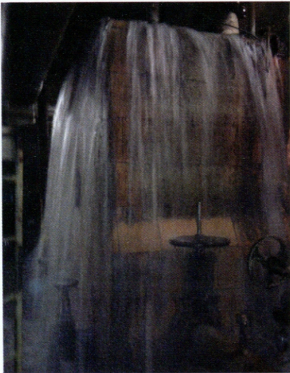
It is tough to keep things dry in any plant when water overflows, such as this one did.
