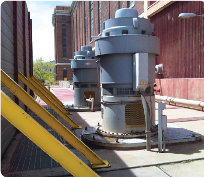
Figure 2: In-service pump motors in Boulder, CO
