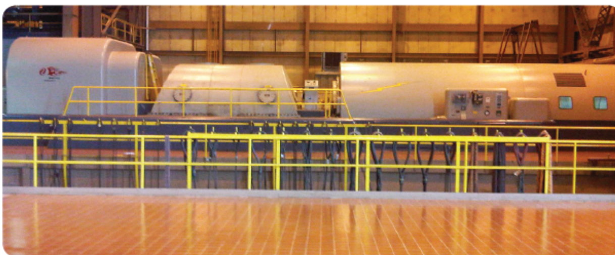
Figure 1: 100MW generator in Boulder, CO
