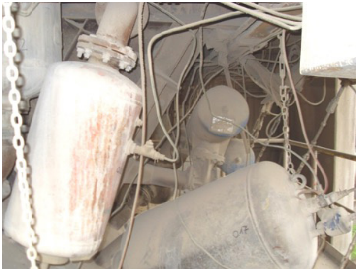
Three different air cannons; all installed incorrectly, and all of which will require frequent maintenance.
