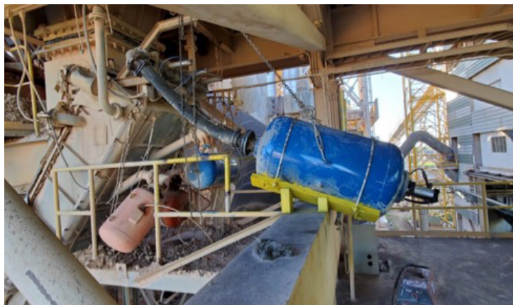
A properly installed air cannon on a material chute. The air cannon is installed close to the discharge points with a high temperature hose which minimises vibration in the chute. This vibration had previously caused many air cannon failures.
