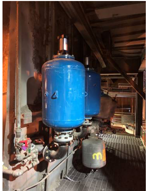
Protecting IGS Air cannons on cooler.
