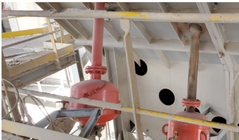
Figure 2. Air cannons should not be pointed upward. This allows easy access for material to enter air cannon and cause failure.
