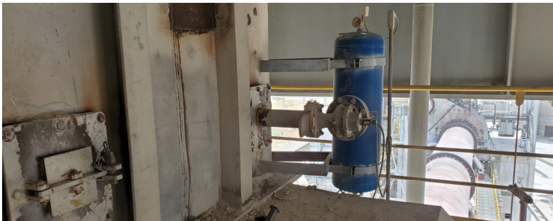
Figure 7. Thermal Safety Shields leak air, allowing false air to enter the tower. Based on 100 air cannons on a tower, the cost of heating this false air is estimated to be as high as US$500 000 per year. Thermal Safety Shields do not protect the air cannon from the process. They protect the workers during maintenance. If you protect the air cannon from the process, maintenance decreases significantly.
