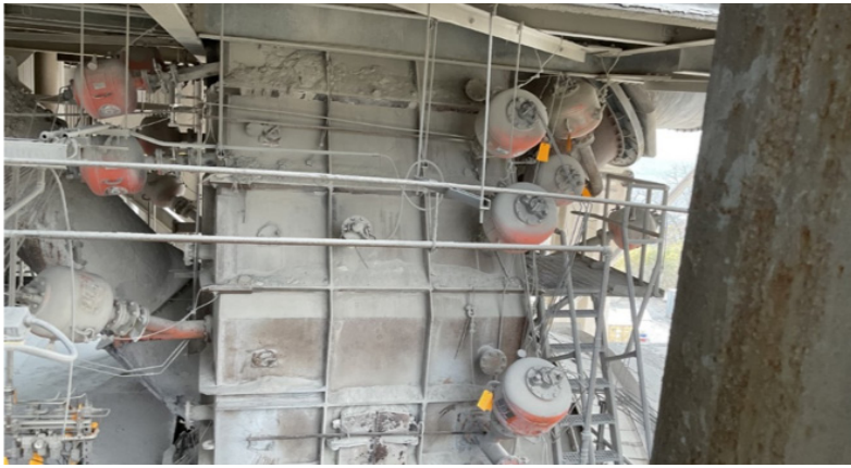
Figure 6. Air cannons that are inaccessible for maintenance fail and cannot be recovered.
