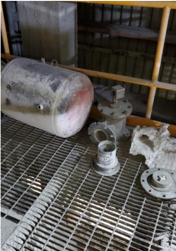
Figure 1. Installation errors are a leading cause of air cannon failure.
