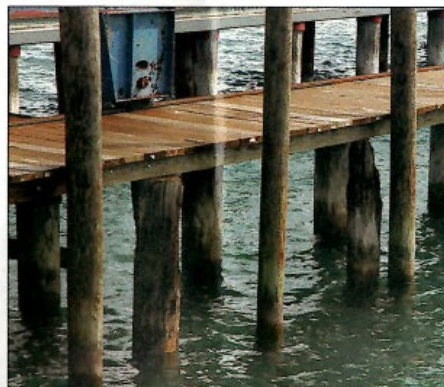
This dock, directly across from the old Tashmoo Park, was built on the original landing site for the Star Lines fleet.
