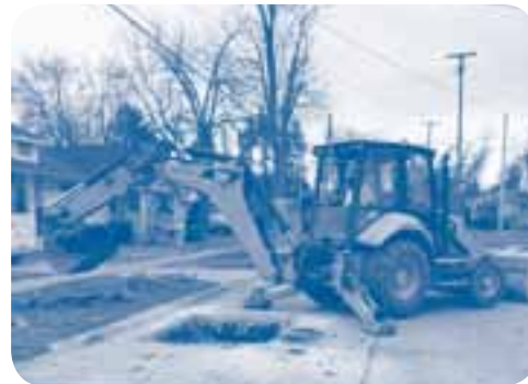
Service line replacement work required by the State's Lead and Copper Rule
