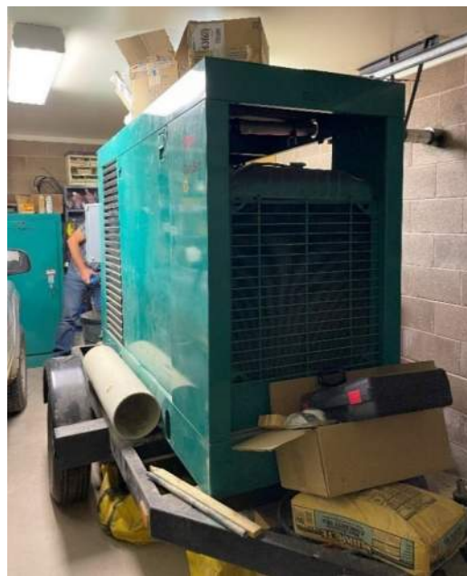
FIGURE 3-10: MAIN LS GENERATOR
