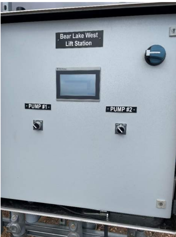
FIGURE 3-25: BLW LS CONTROL PANEL
