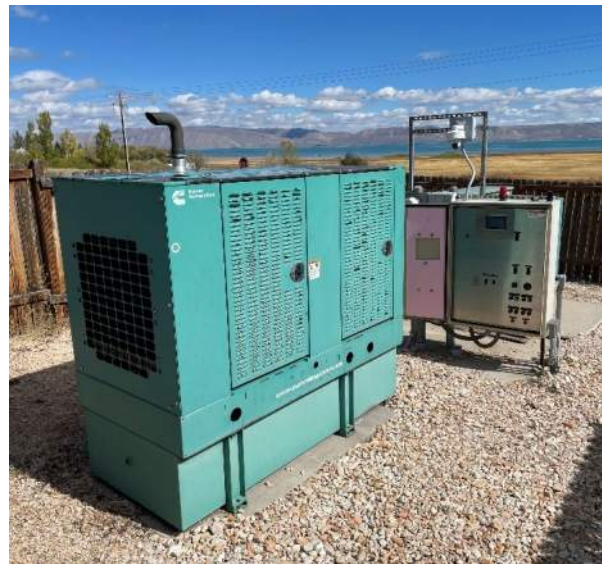
FIGURE 3-14: SOUTH RESERVE LS GENERATOR
