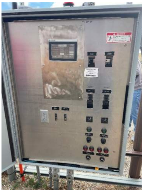
FIGURE 3-21: SUB #9 CONTROL PANEL
