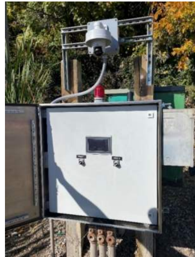
FIGURE 3-4: SOUTH LS CONTROL PANEL
