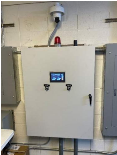
FIGURE 3-9: MAIN LS CONTROL PANEL
