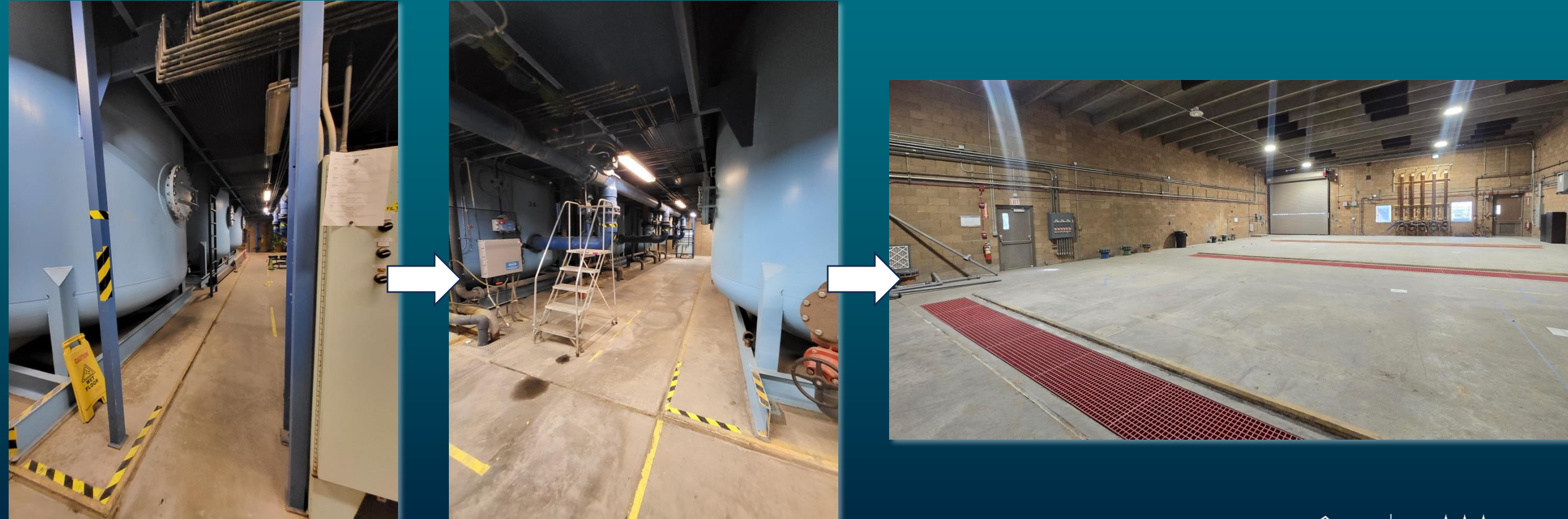
Filter Room Tucson Water's Reclaimed Water Treatment Plant
