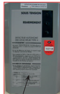
Smoke detecting station
