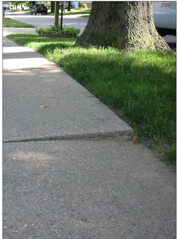
Trees planted in undersized lawn strips can cause sidewalk heaving, creating trip hazards.
