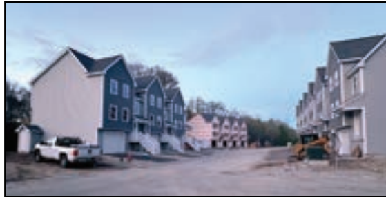
New townhomes being built on Maurais Avenue in South Hooksett. (Tony LaCasse Photo)
