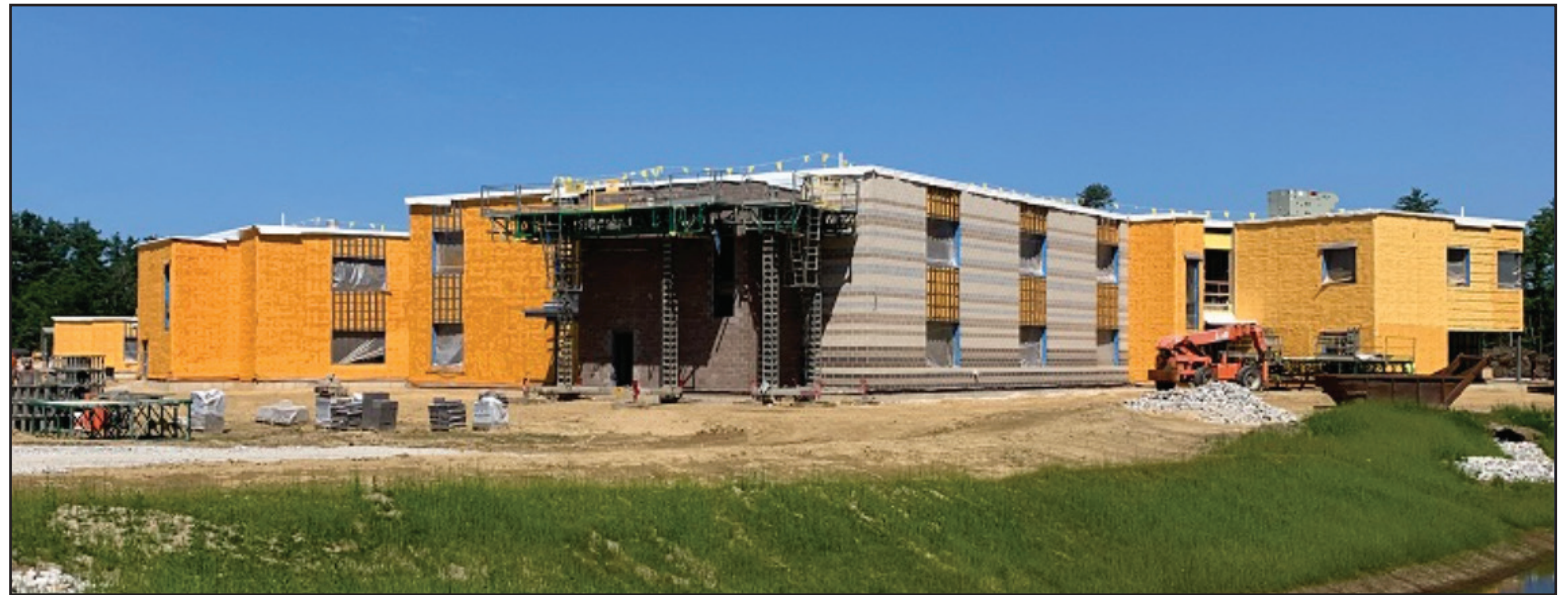
Allenstown's new school is under construction, with students expected to move into the building this spring. (Courtesy photo)
