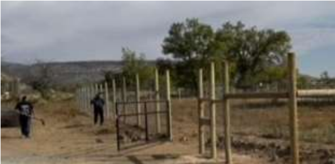
Our guys installing a fence for a community garden in San Fidel
