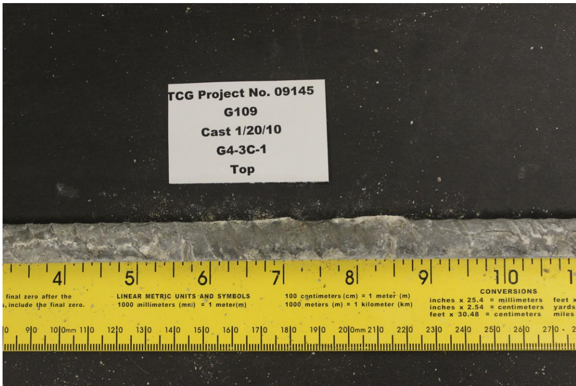
Figure 14 - Top Bar from 2005NS Beam, showing the top surface
