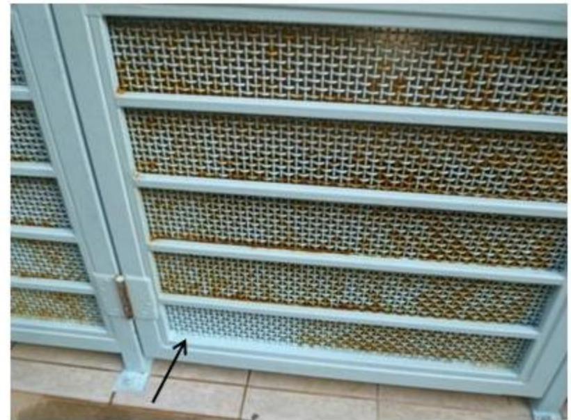
After – unsightly rust staining gone
