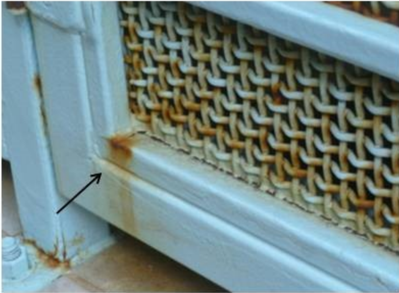
Before – unsightly rust staining
