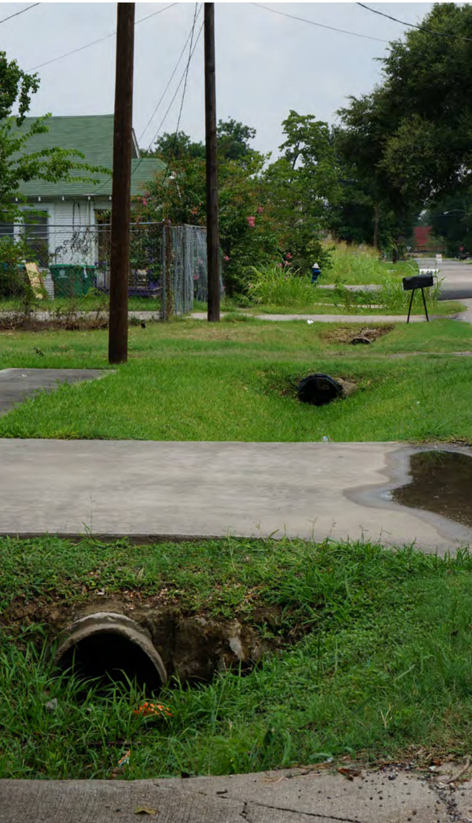
Common storm water management technique used within Houston neighborhoods, to collect water in drainage ditches
