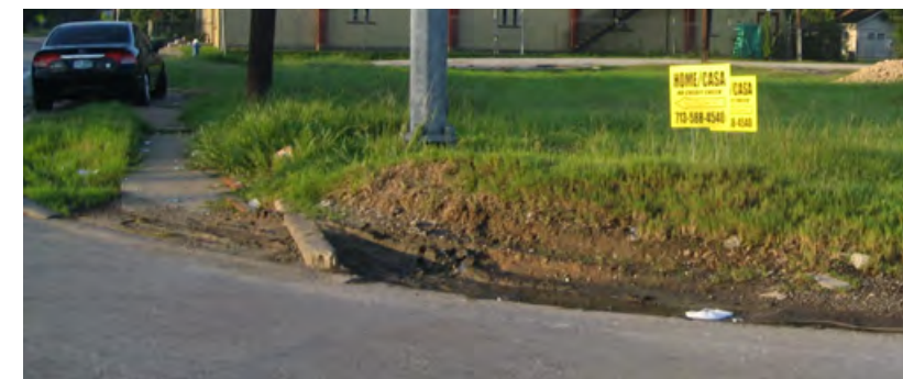
Waco IH-10 Overpass | Non ADA-compliant ramps, poor landscape maintenance
