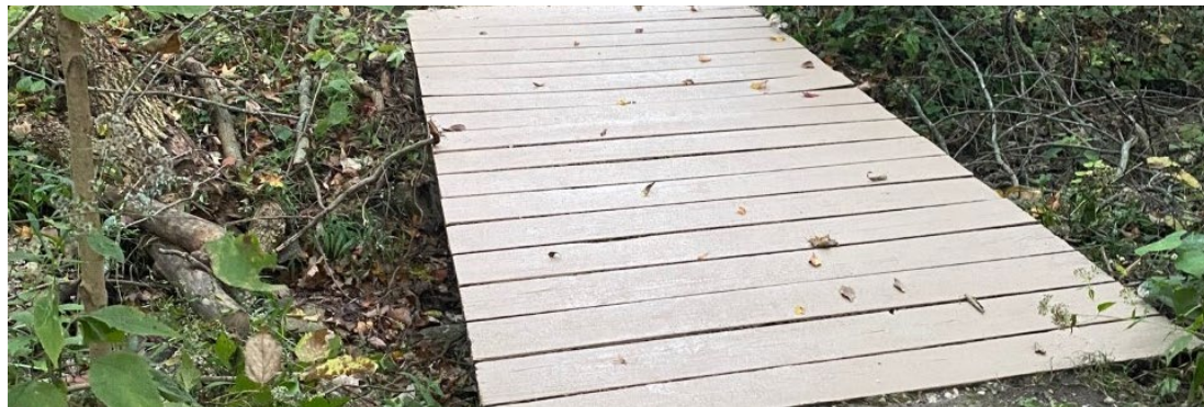
The three bridges throughout the Wildflower Garden received new nonskid surfaces. This new surface is an extra safety feature to visitors on days the bridge is wet due to weather.
