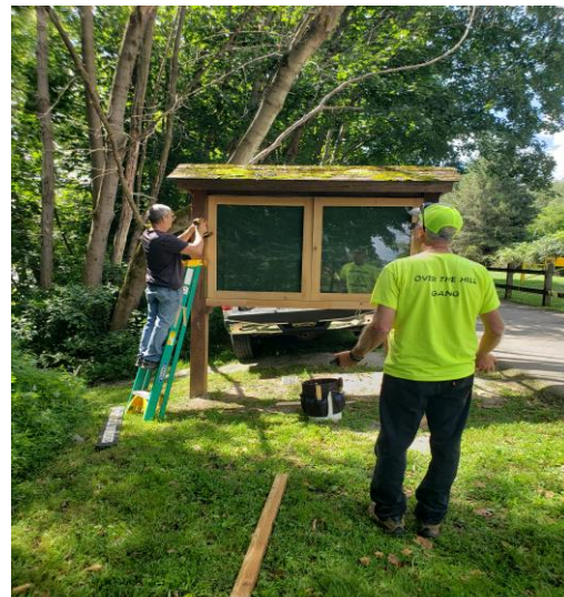
Scott Shoff installing new doors on one of the info kiosks, Bert Condie assisting
