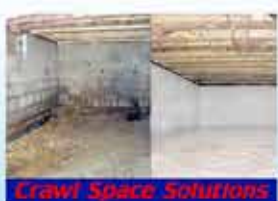
Crawl Space Solutions
