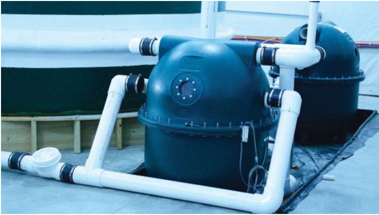
AST PolyGeysers Bead Filters were selected as a key component of the indoor recirculating aquaculture system
