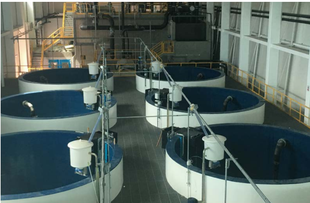
AQQUUA Recirculating aquaculture farm in Thailand.
