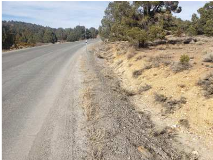
The Drainage Ditches are maintained through the Operating Budget. An allowance for major repairs has been included in the Reserve Study to be used if needed.
