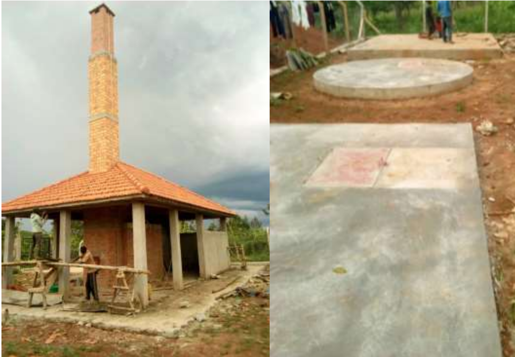
Status of the project by end of April 2022 (Left: Incinerator; Right: Waste Pits)
