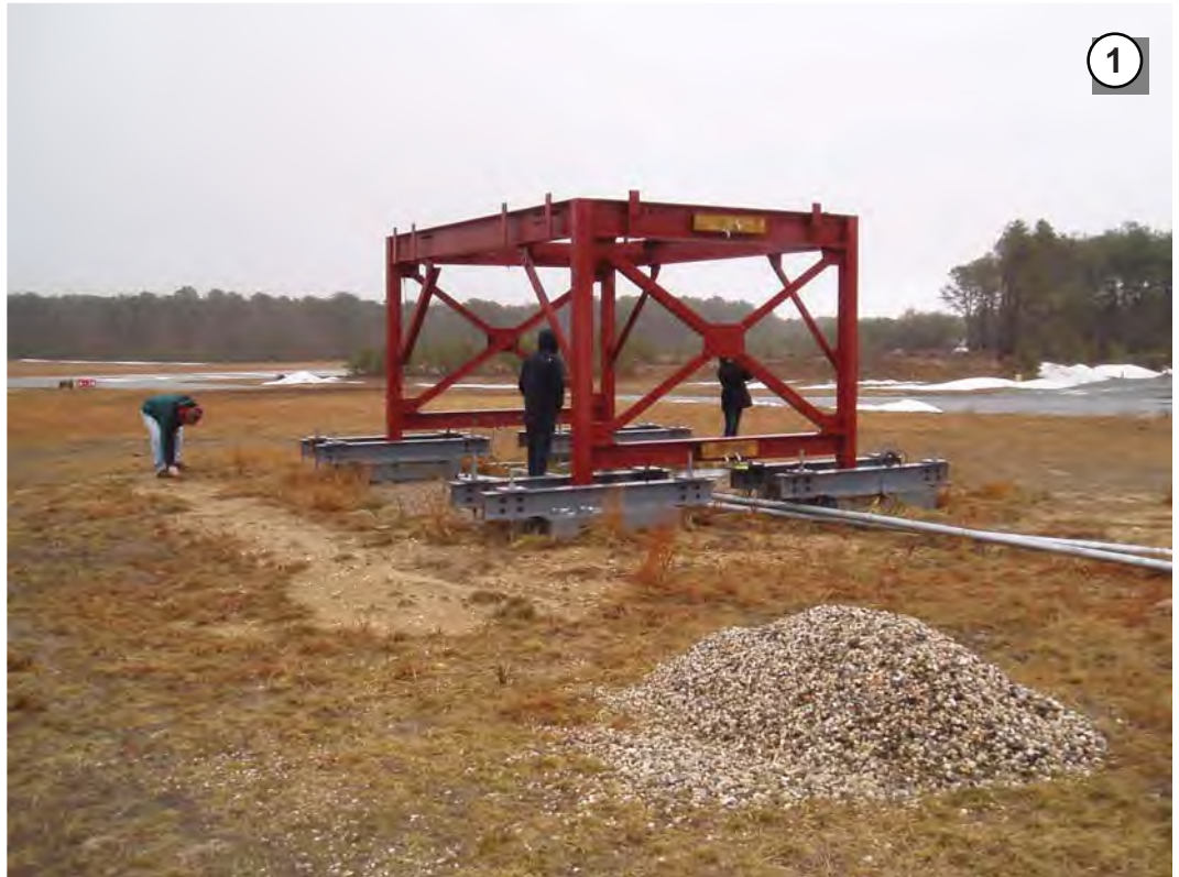
Looking east/southeast at the footings and the support structure of the mobile ATCT installed at the Preferred Alternative in 2012 (Field Photograph P1010005, February 27, 2013).
