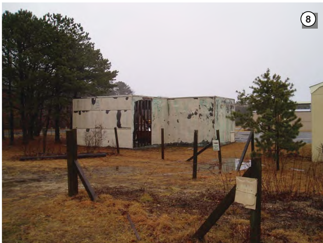
Looking south at Building 7 which was being dismantled in February 2013. (Field Photograph P1010003, February 27, 2013).
