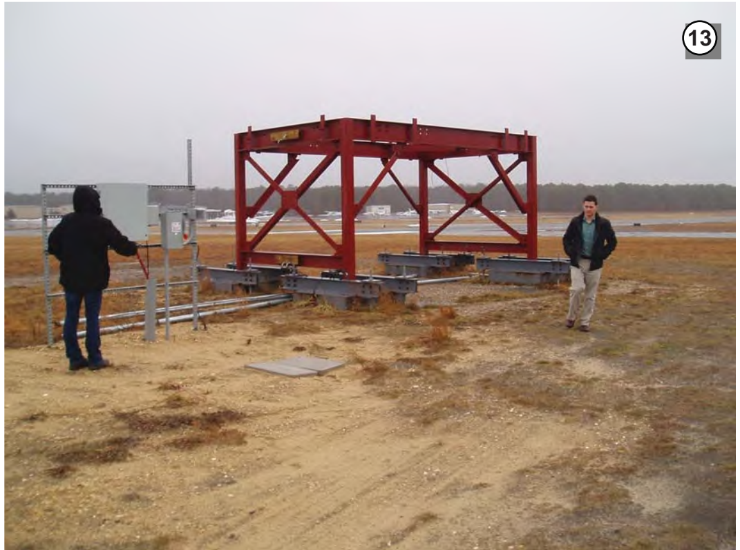
Looking northeast at the mobile ATCT footings and support structure. The Airport terminal building complex is in the background (Field Photograph P1010006, February 27, 2013).
