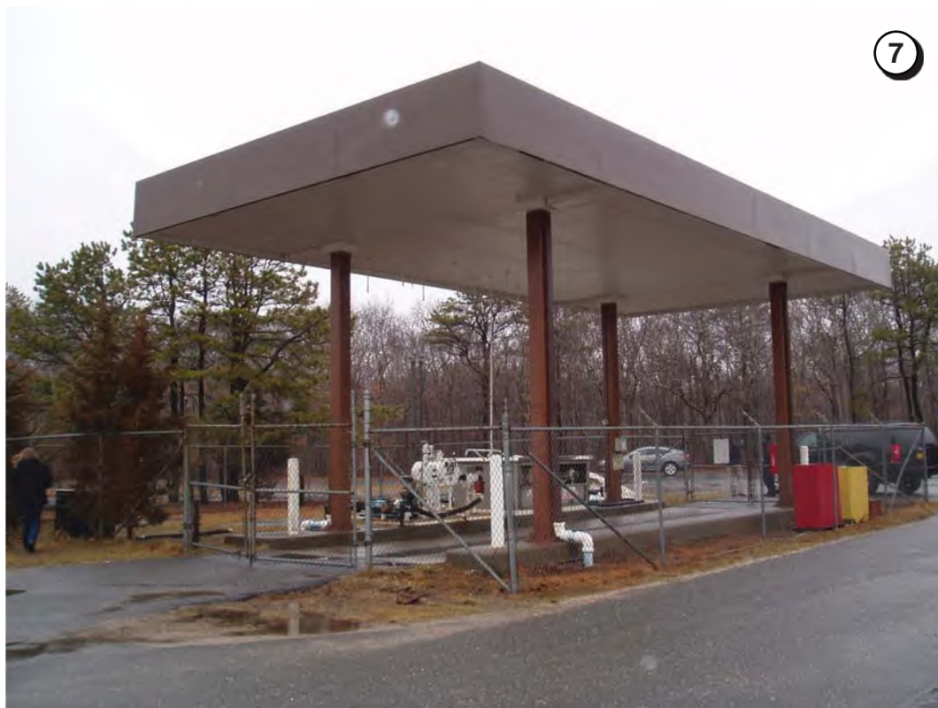
Looking northeast at the Airport fuel farm adjacent to Daniels Hole Road. (Field Photograph P1010002, February 27, 2013).
