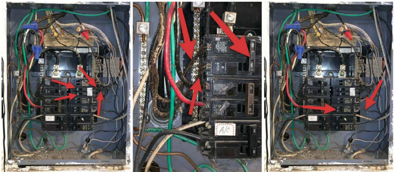
30 amp breaker utilizing 14 AWG wiring on two circuit breakers, significantly undersized conductor which is a potential safety hazard.
