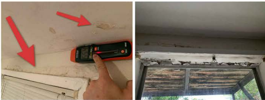
Moisture was over 55% around window
