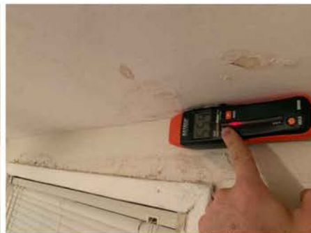
Moisture was over 55%, which is conducive to mold growth.
