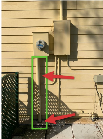
Service entrance from underground Southeast
