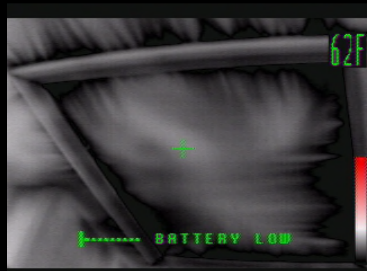
Air leaking around attic hatch.
