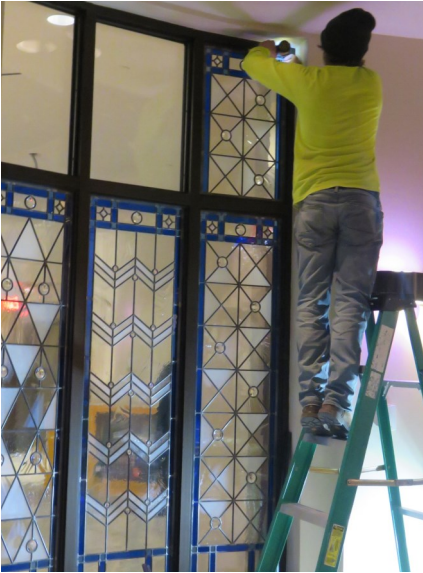
Installation of the new stained glass by the baptismal font, thanks to several generous donors.
