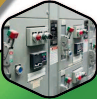
Switchgear & Motor Control Centers (MCCs)
