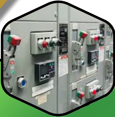
Switchgear & Motor Control Centers (MCCs)
