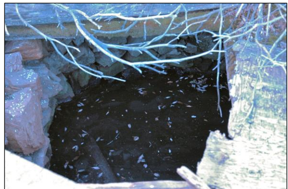
Figure 15. Example of an improperly abandoned well.
