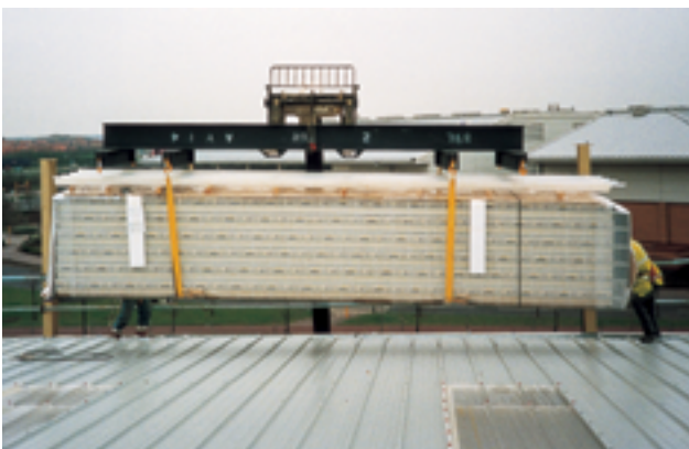
Figure 31 (above) Delivering sheets to roof level onto the completed load-bearing section and behind the leading edge (note that the roof lights include mesh protection and are non-fragile)
