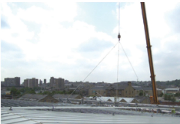
Figure 36 (a)–(c) 24-m long roof panels being mechanically lifted from ground level and installed on roof
