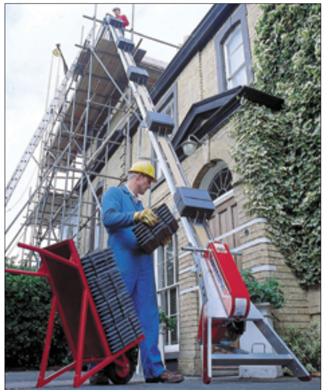
Figure 4(b) Domestic hoist
