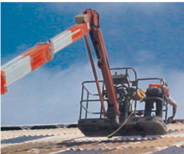
Figure 15 A mobile elevating work platform being used to replace a roof sheet
