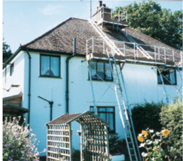
Figure 25 Proprietary system for access to roof and chimney
