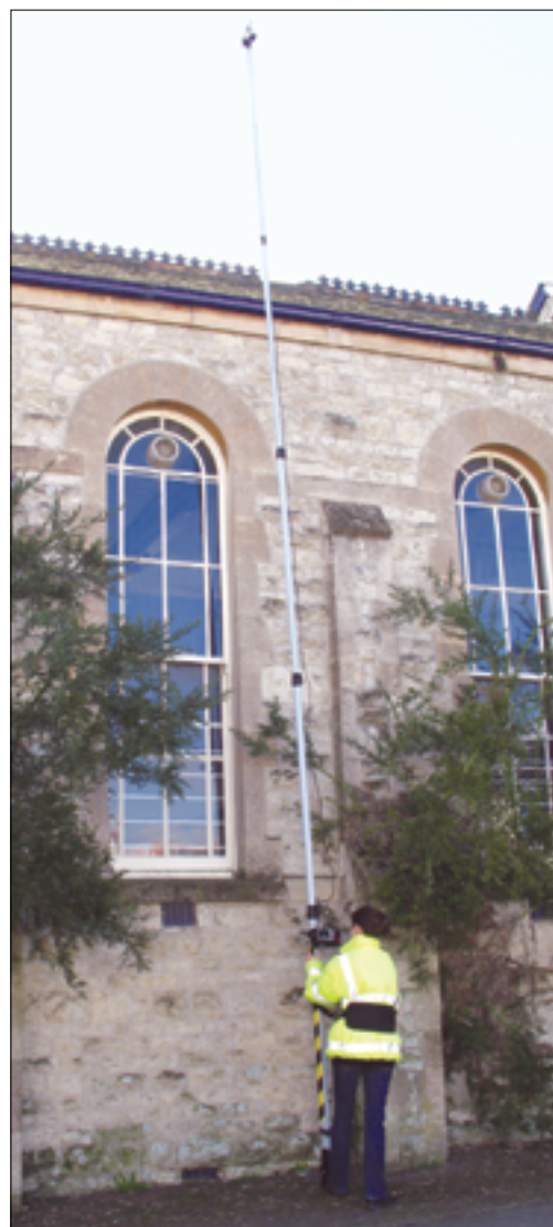
Figure 10 Remote inspection mast with hand-held lightweight CCTV system (image courtesy of Survey Support Ltd)
