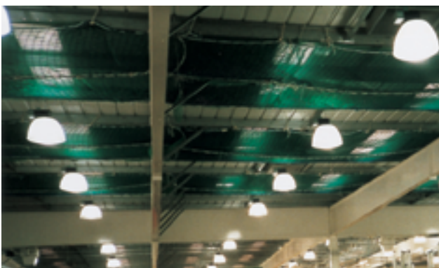
Figure 28 Safety netting used to minimise the distance and consequences of a fall for roof lights during roof works
