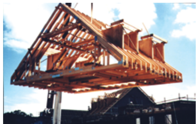
Figure 21 Craning a pre-assembled roof into position greatly reduces the need for work at height (image courtesy of the Trussed Rafter Association)
