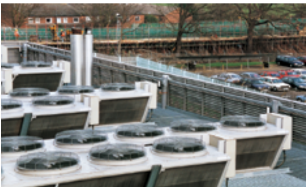
Figure 39 Parapet edge protection included as an integral design feature
