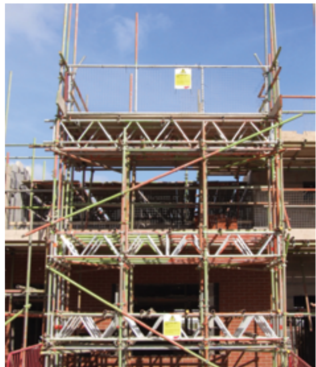
Figure 32 (right) Loading bays should be designed for the actual weight of the materials to be placed on them and include an additional allowance for impact loads from mechanical handling (eg cranes or forklifts). A notice should clearly display the safe working load
