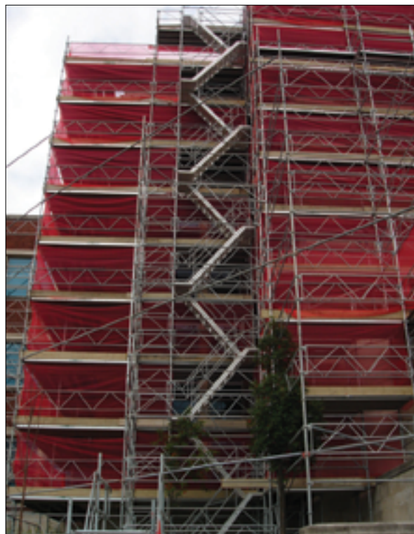
Figure 3 Stair towers provide good access. Make sure they are properly secured and erected (image courtesy of Turner Access)
