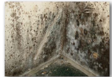
Water Damage & Mold in Wood Home
