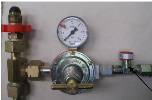
Left: Bottle connector regulator valve pressure gauge and excess flow safety valve
