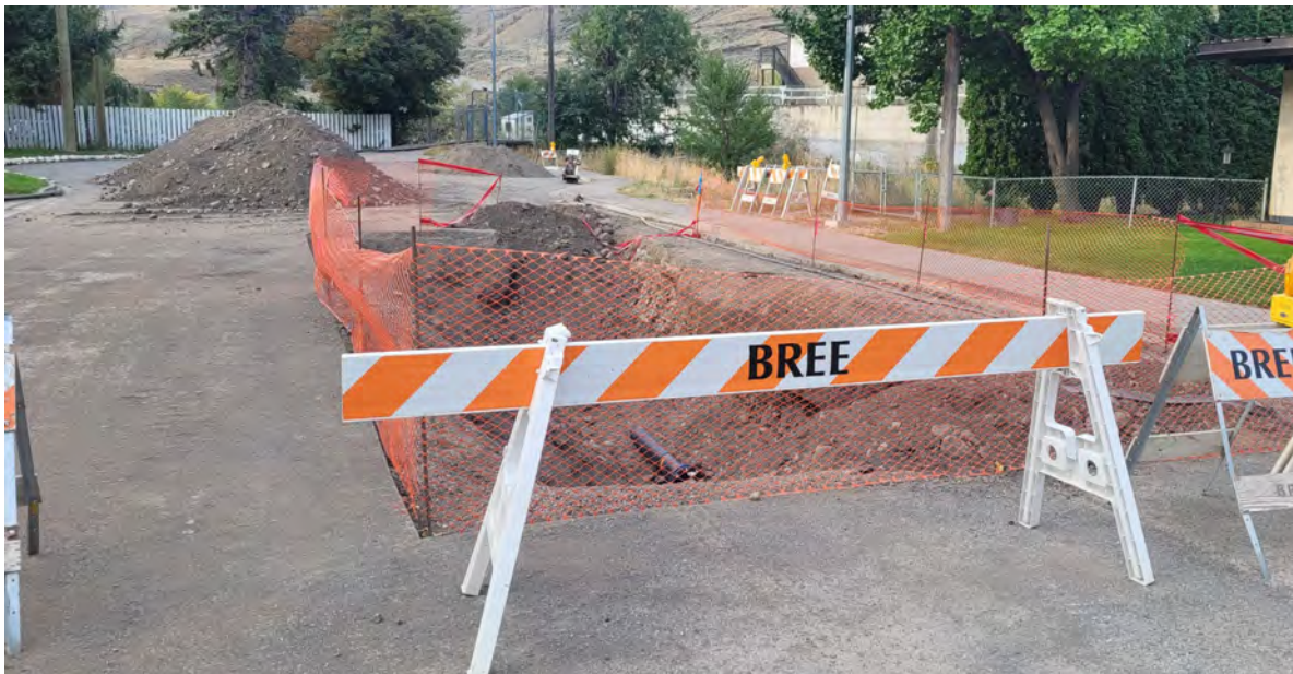
Photo of Phase 3 excavation for new water crossing at Collins Road. Directional drilling was used to avoid working within the waterway.
