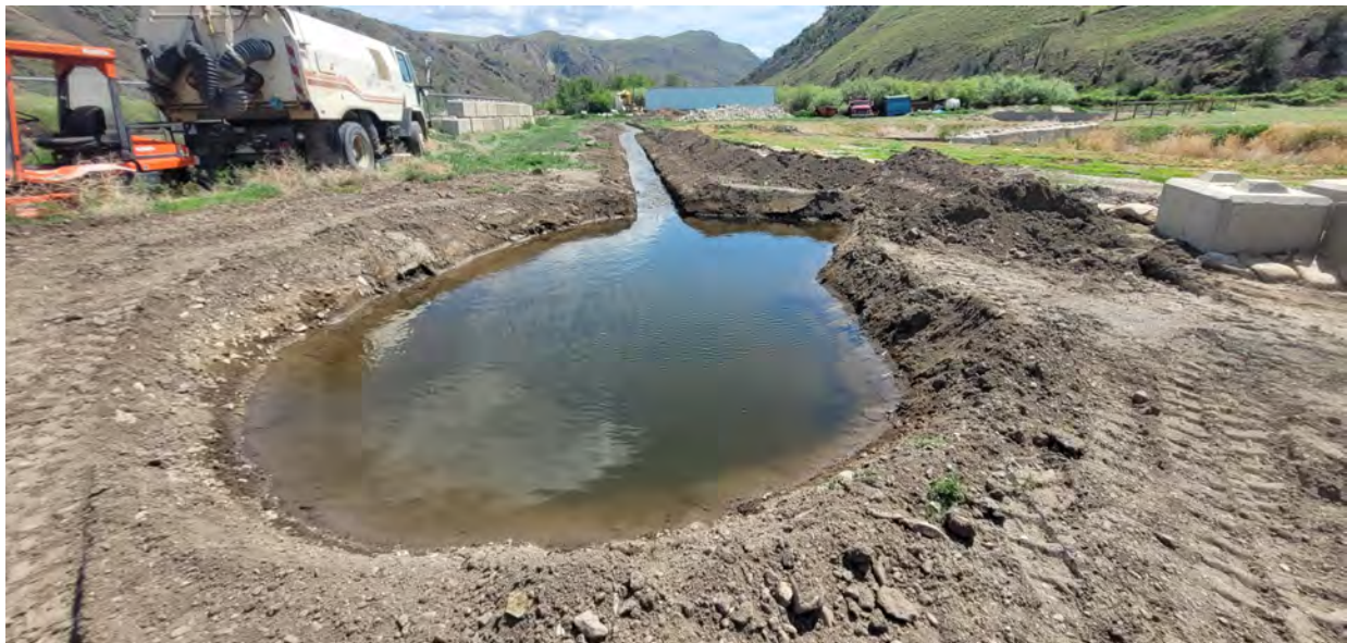
Photo of Wastewater Treatment Plant outfall after excavation. The final stage of the treatment process sees the treated effluent return to the waterway.
