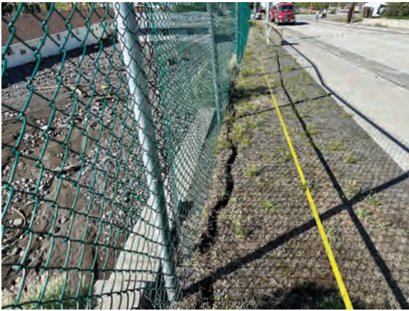
Figure 2: Crack above wall (looking southwest)
