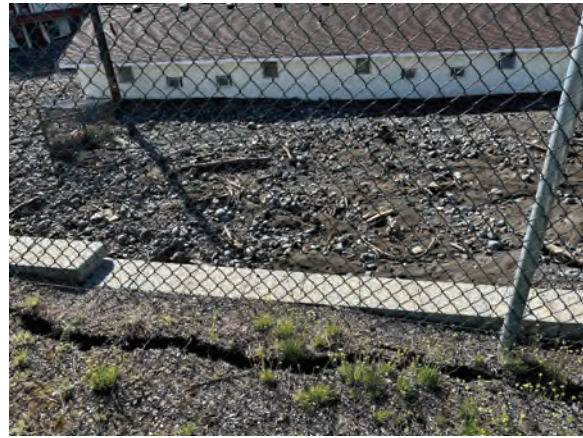
Figure 3: Crack above wall (looking southeast)
