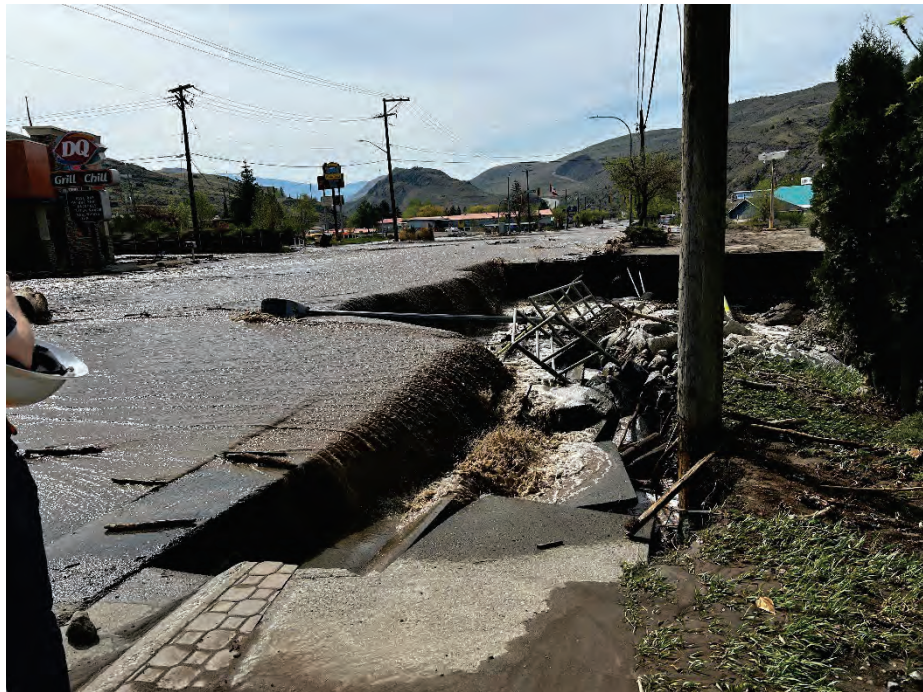
FIGURE 1-3: HIGHWAY 97 EROSION FROM OVERLAND FLOW (MAY 04, 2023)
