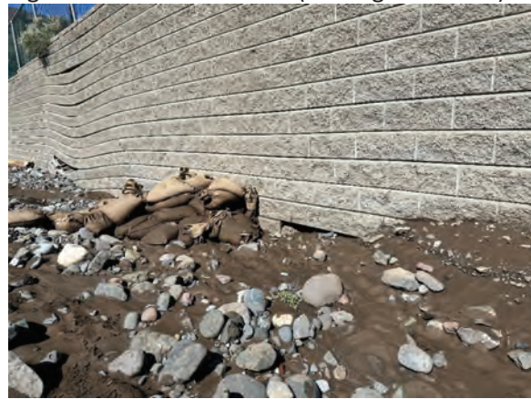
Figure 5: Wall failure (looking southwest)
