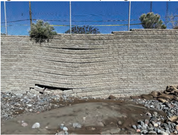
Figure 4: Wall failure (looking northwest)
