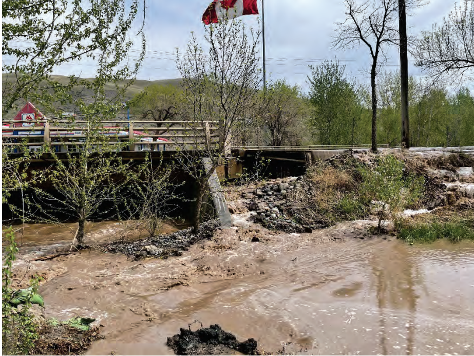
FIGURE 1-2: EROSION BEHIND TCH BRIDGE ABUTMENT (MAY 03, 2023)
